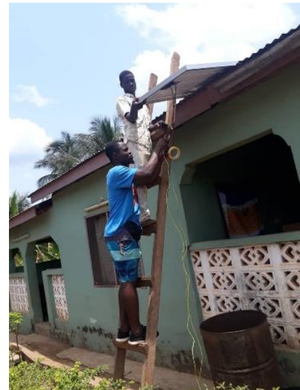
Figure 1. Emmanuel and Kojo-Nkwanta resident installing a solar panel for an ISEC cooker.
