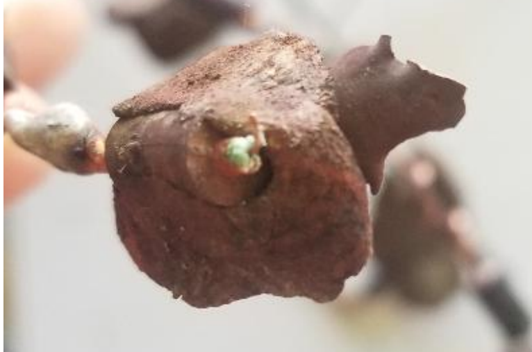
Figure 1. Corroded diode lead of a cooker constructed by twisting all connections. Surrounding the diode is erythritol and JB weld. During construction, diode bodies were glued to the pot using JB weld, but leads were left uncoated.
